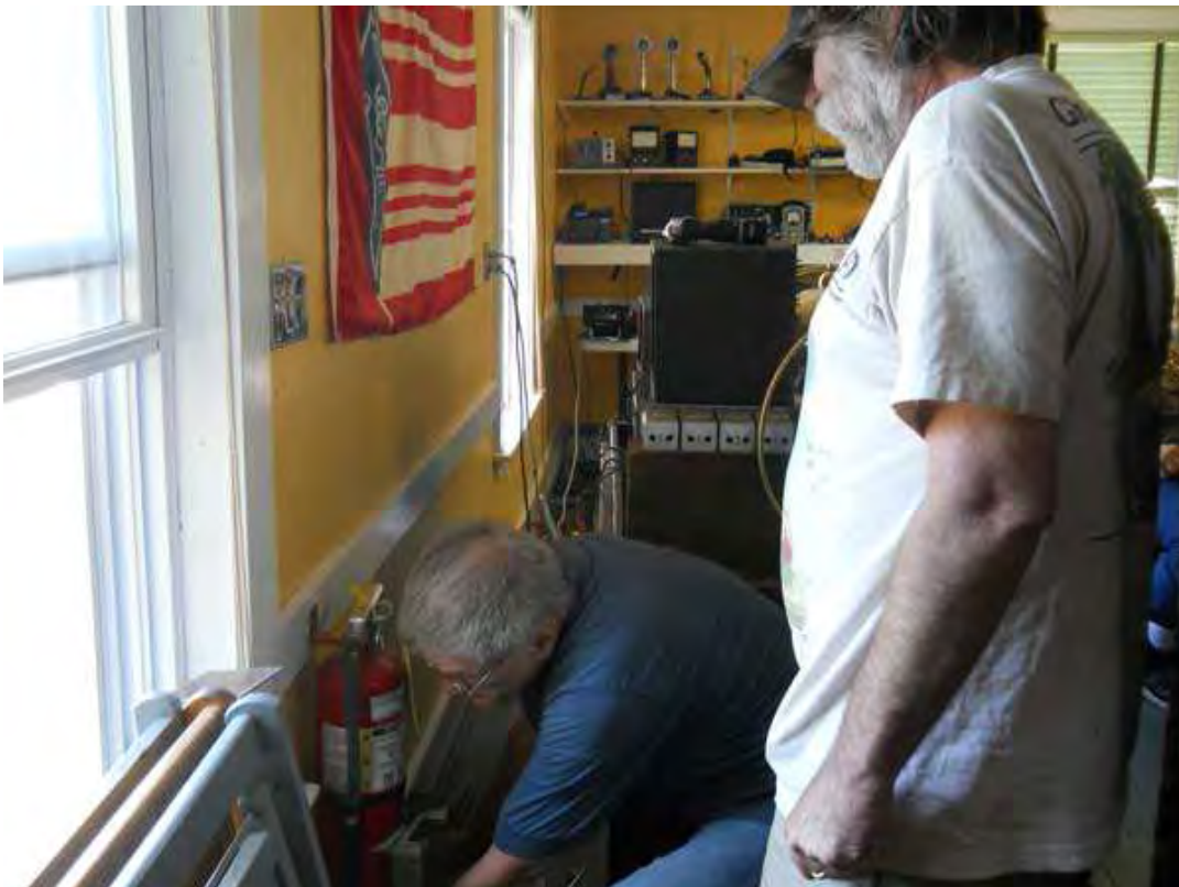
Dick K1VRA and Jake K1LDL install the runner for the new electric wiring on the second floor of the clubhouse
