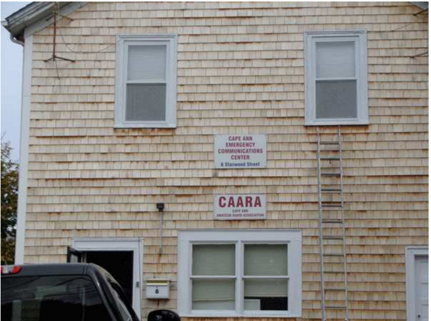
Your House Committee at work: Ross on the ladder scraping, caulking, and painting the second floor windows.
